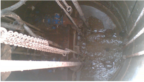
A typical wet well application where Quantum 2 is used for Pump Control.
